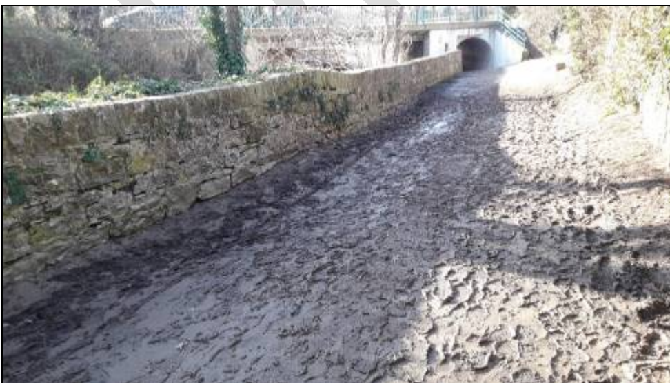
Figure 16: Wall on Left bank from A525 to Brookhouse Mill. Crack in wall potential seepage routes Source: NRW
