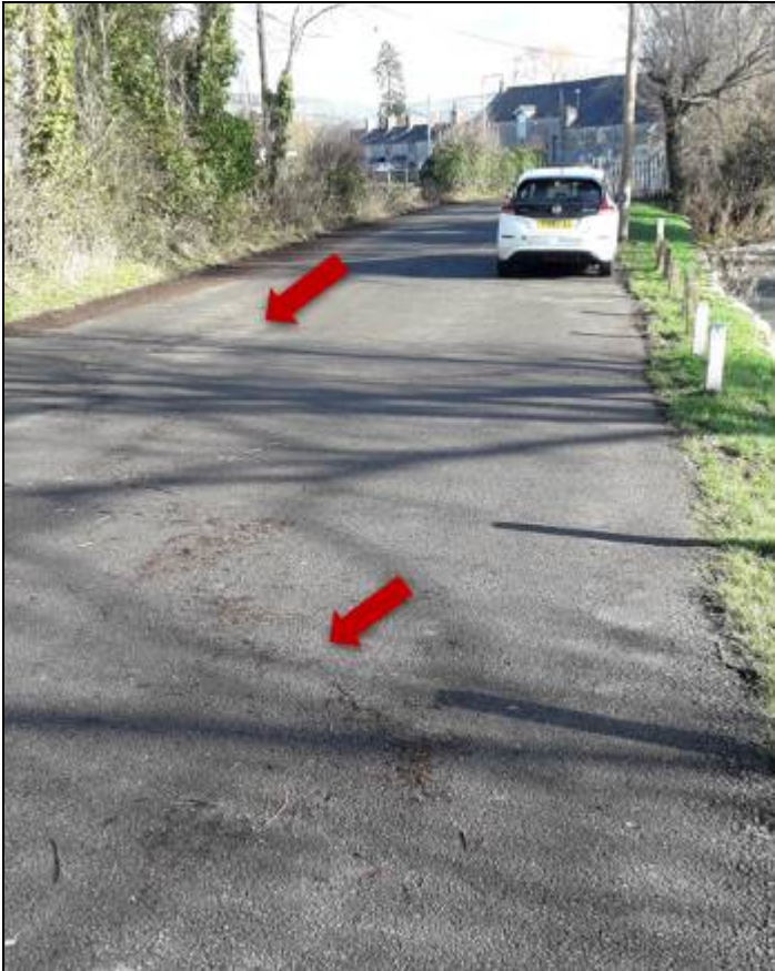
Figure 10: Photo of wrack mark left by Afon Ystrad on Brookhouse Road adjacent to right bank by weir at small layby. Source: NRW
