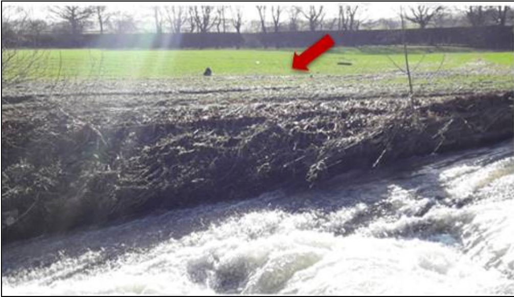
Figure 9: Photo of wrack mark left by Afon Ystrad on Right Bank just downstream of the weir 12 February 2020. Source: NRW
